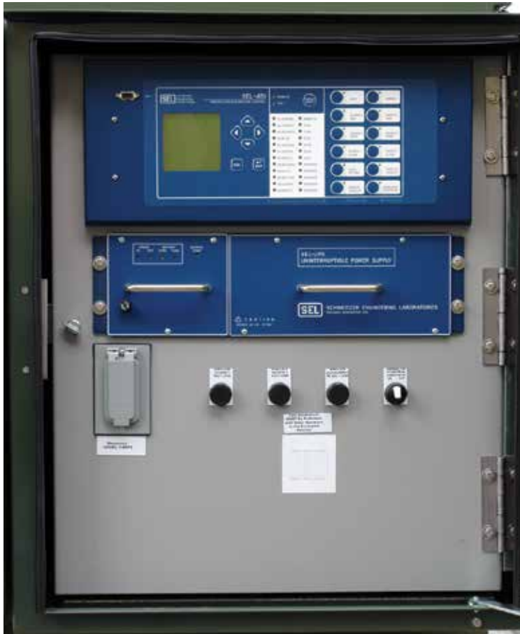
Figure 1. View of typical low-voltage control cabinet (above) that includes the automatic-transfer control relay and associated components.
