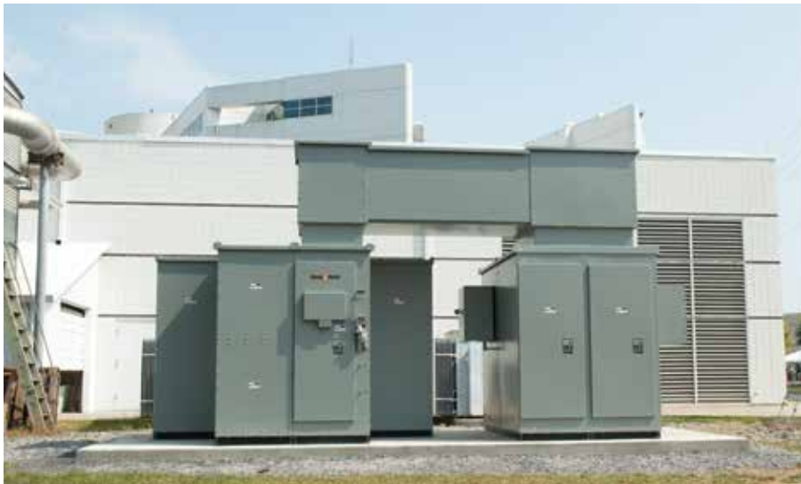
Figure 3. Automatic-transfer switchgear with Fast-Trip Transfer motor operators is pictured in the photo above. Transfer to the alternate source is achieved in approximately twenty (20) cycles.
