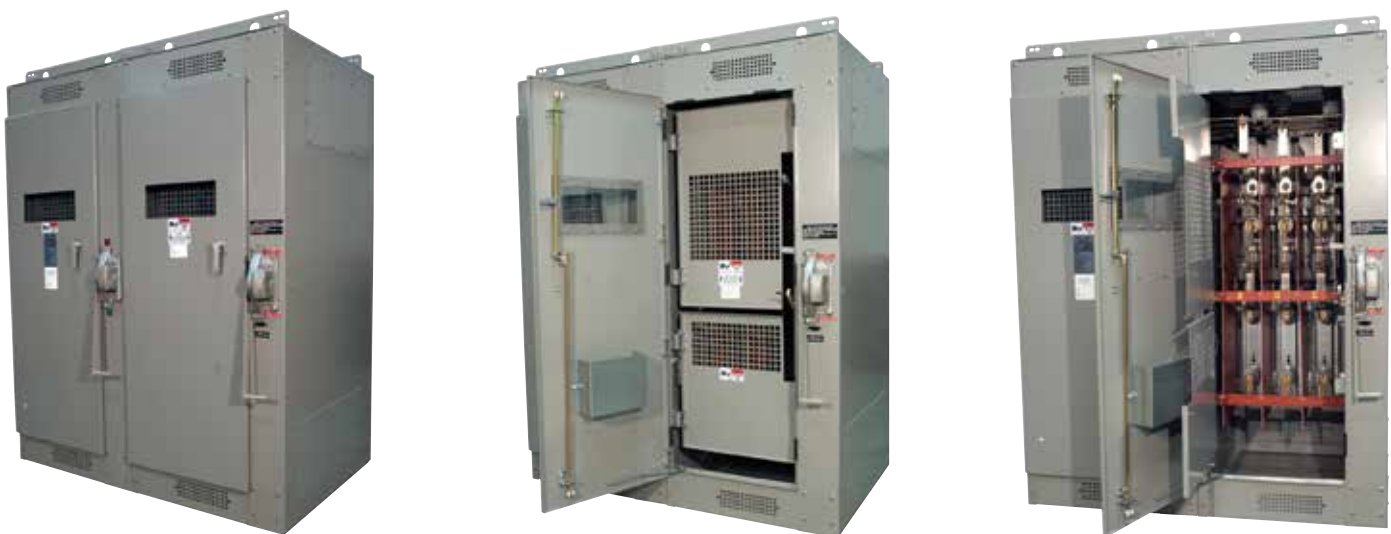
Pictured above are typical feeder bays with automatic-trip (shunt-trip) switches, providing feeder isolation when a single-phase condition (such as a blown feeder fuse) occurs.
