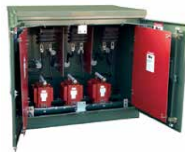
Metering Transformer Compartment With Barriers Secured Open
