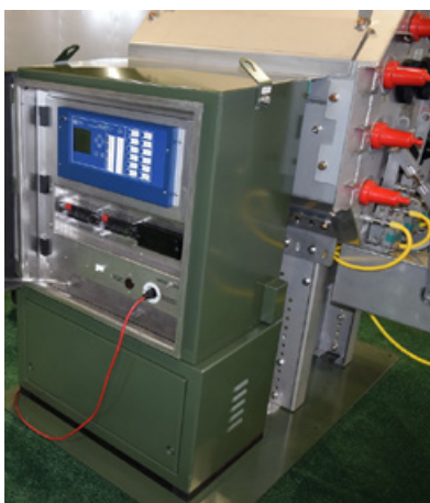
Figure 10. Schweitzer Engineering Laboratories SEL-451 integrated in exterior cabinet.
