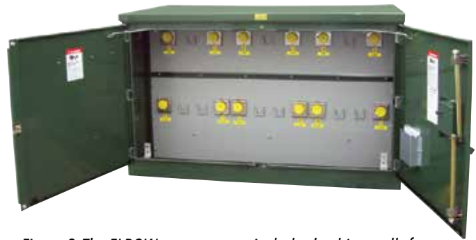
Figure 2. The ELBOW compartment includes bushing wells for connection of (the normally customer furnished) inserts and elbows. At the top are the bushing wells for the incoming (source) circuit connections with an IN and OUT position for each phase and a parking stand between them. At the bottom are the bushing wells for the outgoing (load) circuit connections (two fuses per phase) and a parking stand is provided for each outgoing circuit.
