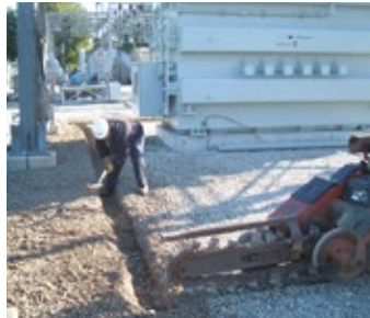
Dike installation for oil and rainfall requirements.
